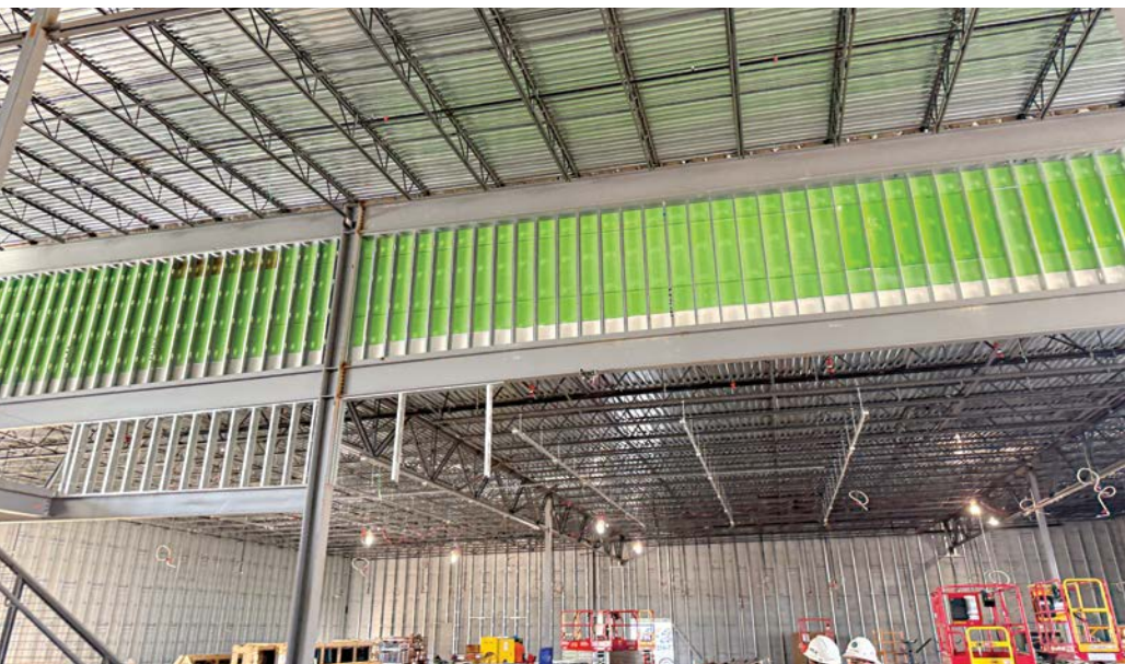
The design for the 2,229.7 m 2 (24,000 sf) WOW! Entertainment Center in Fenton, Mo., includes infrastructure for dining and recreation, and uses steel-framed bar joists and joist girders for a strong, high-performing roof.
