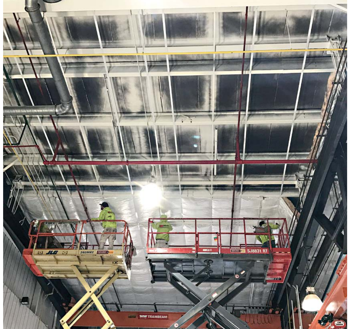
Involving insulation partners early in the design process promotes strong choices that ensure metal buildings preserve their functionality and appearance.
