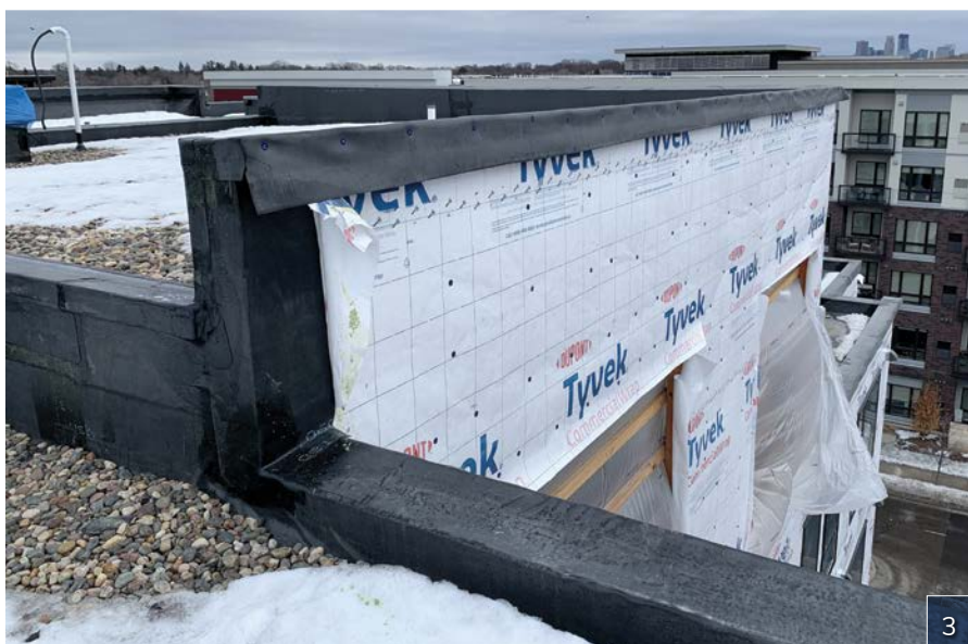
Photo 1: Out-of-sequence roof-to-wall work interrupts air barrier continuity before the transition membrane is installed.
