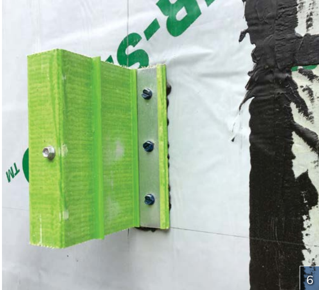
Photo 6: Sealing metal wall panel clip fasteners adds critical protection at unavoidable air barrier penetrations.
